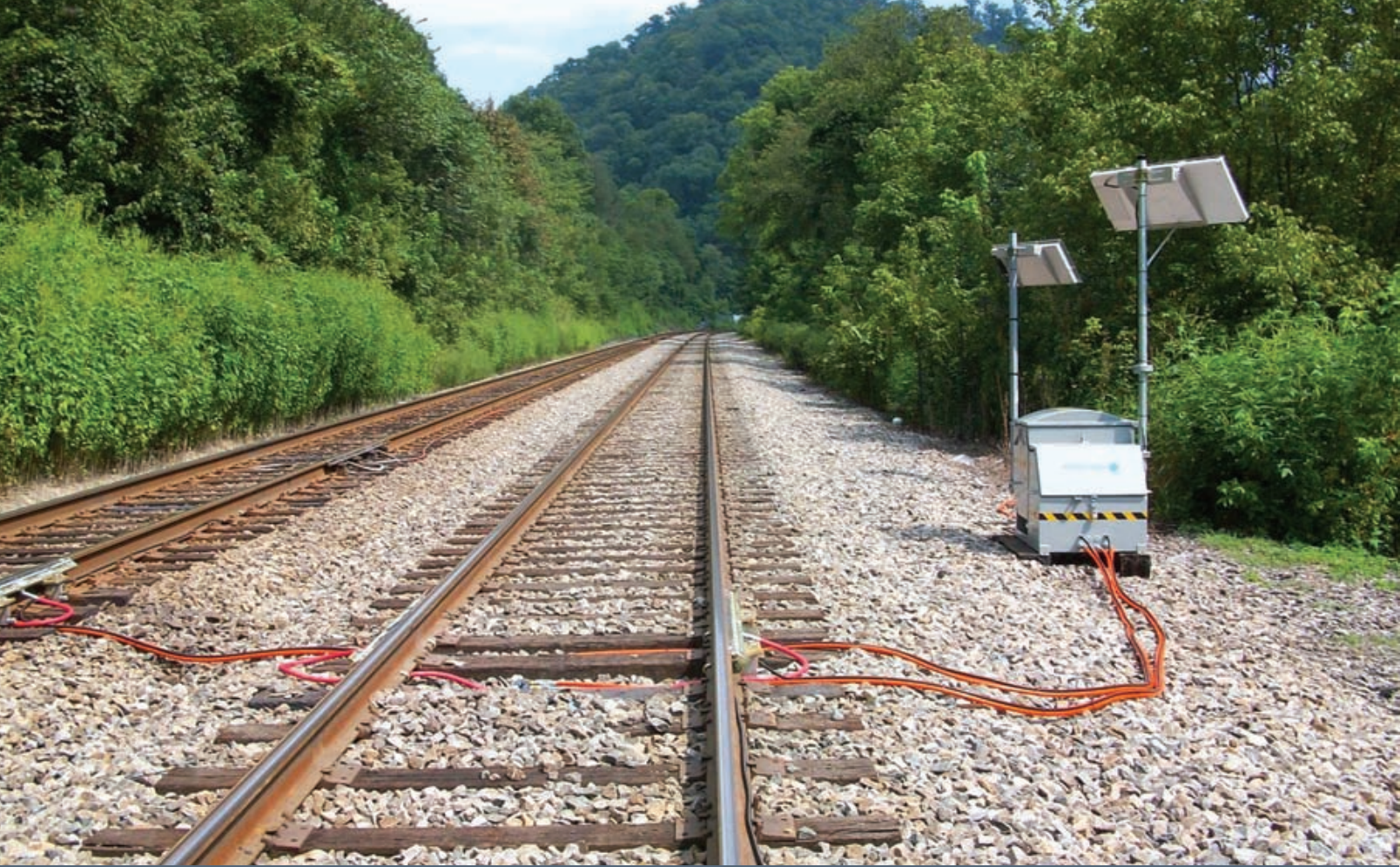
▲ WAYSIDE FRICTION MANAGEMENT SYSTEM INSTALLATION
