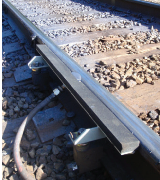
Top of rail foam bar friction management system applies KELTRACK rail lubricant
