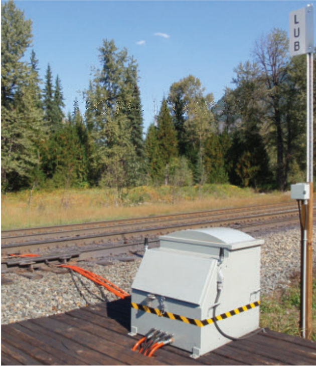
Remote notification activates PROTECTOR rail lubricator to apply friction modifier to track
