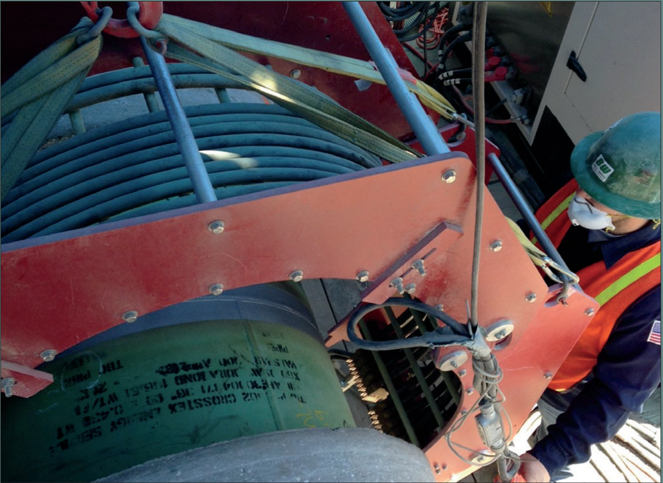
L.B. Foster Ball Winch Field Services team provides state-of-the-art joint coating for infield pipeline construction.
